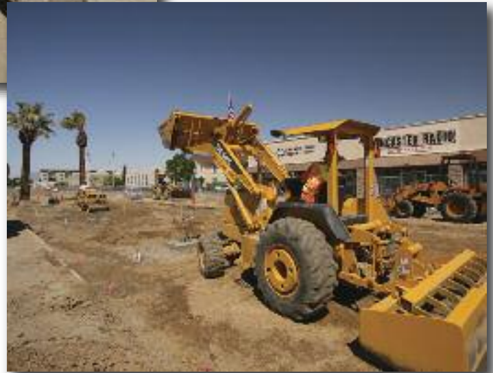
Workers are busily transforming vision into reality. The brick paved medians will be lined with trees creating a shaded canopy.
