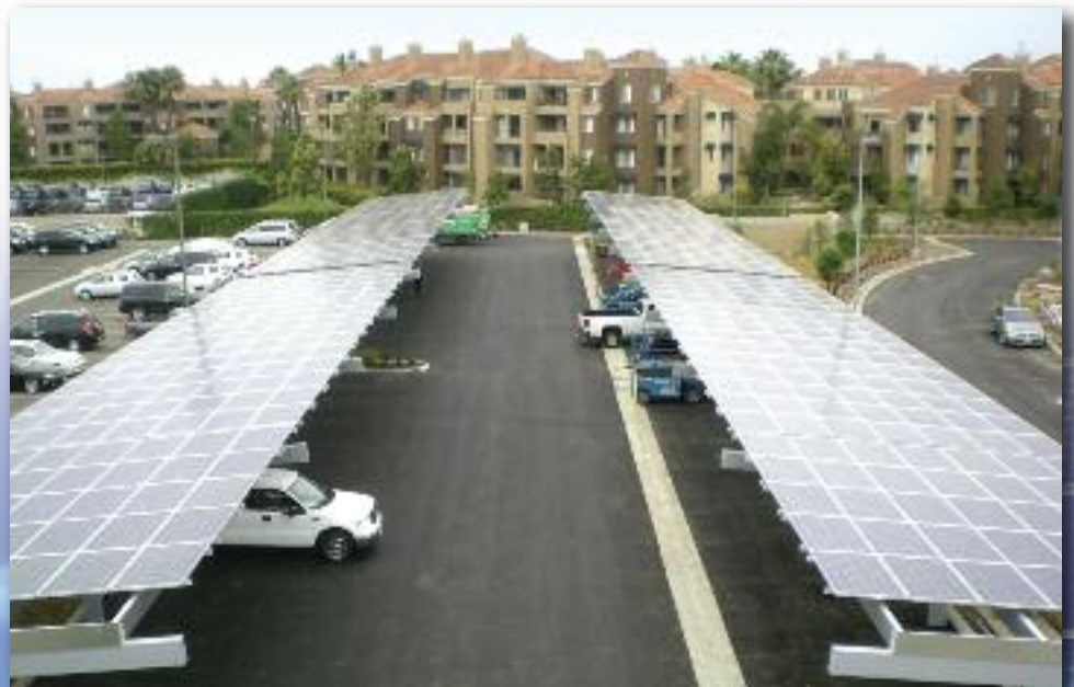
SolarCity solar carport installation at Coast Community College in Costa Mesa, CA
