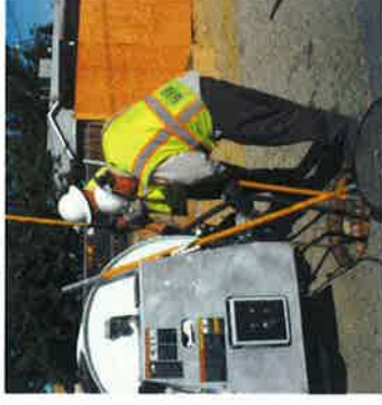
Utility workers operating a jetting machine to clean grease and clear flushable wipes from sewer pipes
