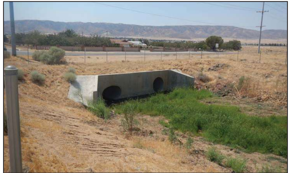
View of concrete culvert located at the southern boundary of the Avanti South parcel.
