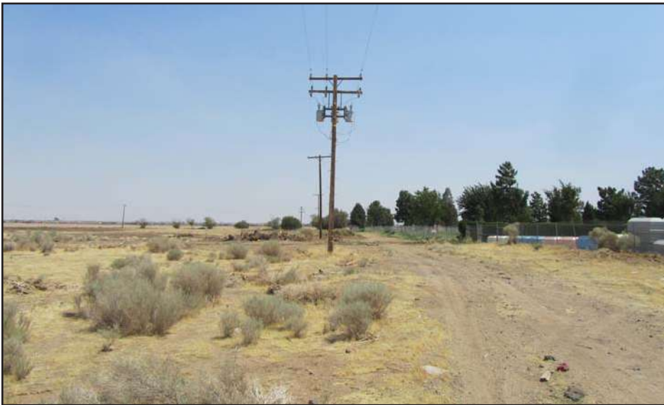
View of on-site transformer along the southern boundary of the Avanti West parcel.
