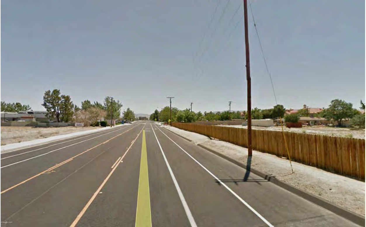
Picture 27 - 15th Street West, Avenue K-8 to Avenue K-11. No Sidewalk
