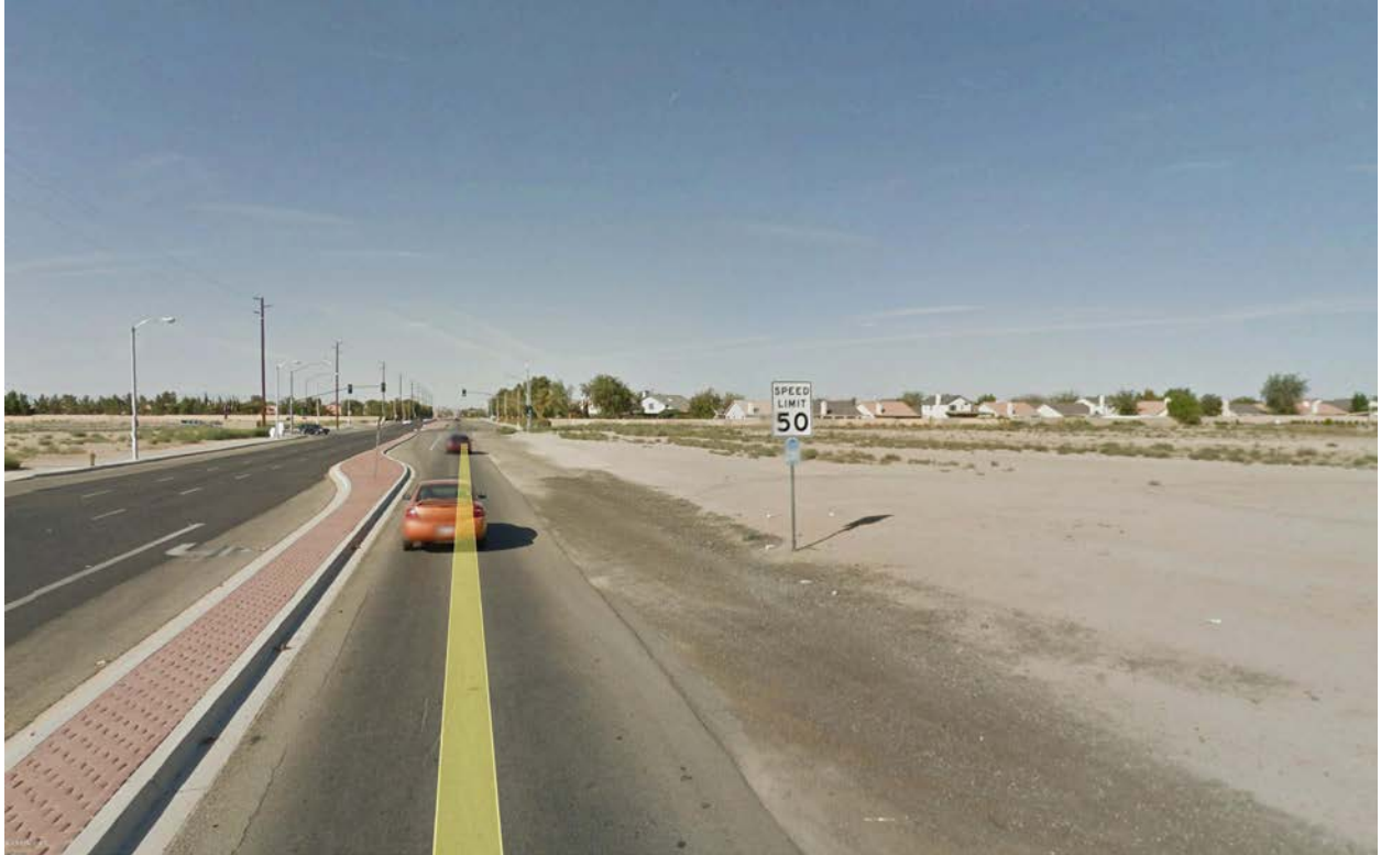
Picture 35 - 20th Street East, Lancaster Blvd to Avenue J. No Sidewalk, Curb and Gutter. Bus Stop is in the Unpaved Shoulder
