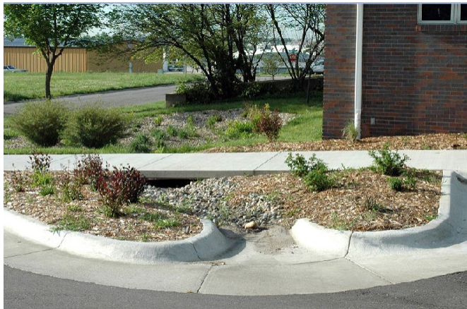
A bulb-out containing a swale with access to street runoff.
