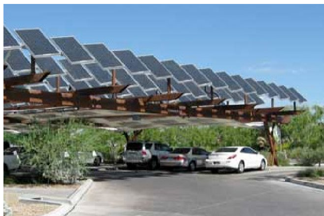
A grid of solar panels with fabric shades over a parking lot.
