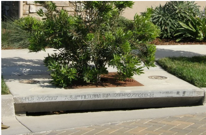
Storm drain filter systems help to naturally filter runoff.
