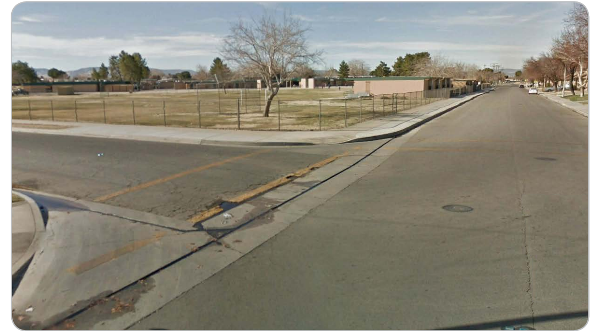
Kettering Street & Rodin Avenue Westbound Lack of high visibility crosswalks, stop signs, and stop lines.
