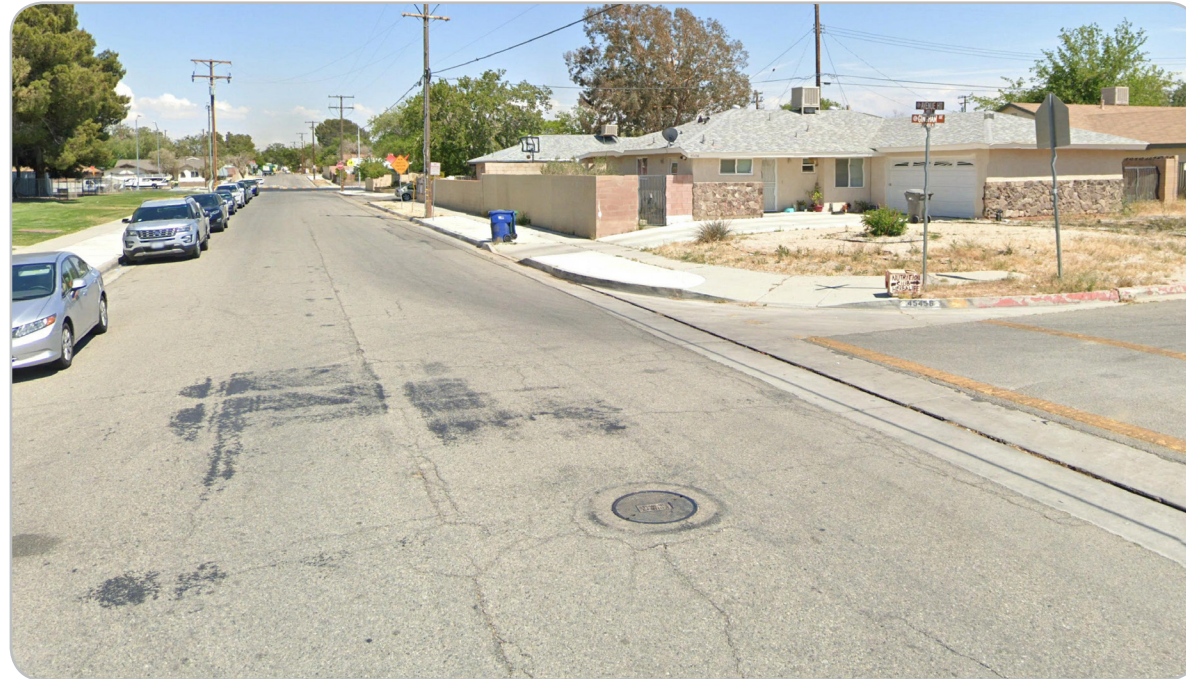
Avenue H11 & Gingham Avenue eastbound Lack of high visibility crosswalks, stop sign, stop line, advance yield line, and sidewalk.
