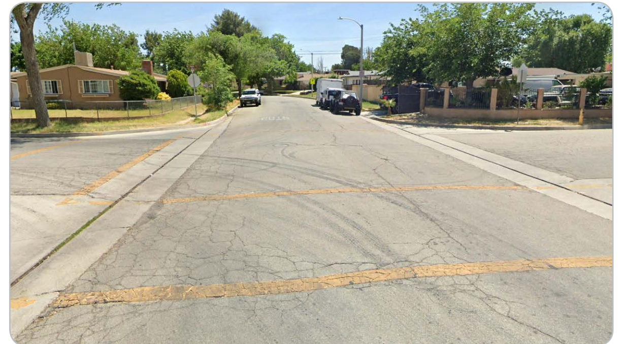
Nugent Street & Foxton Avenue southbound Lack of high visibility crosswalks, advance yield lines, stop lines, and sidewalks.
