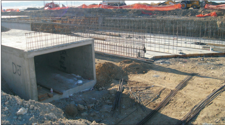
Photograph 1: Looking west from the northeast corner of West Ave. J and 65 street at recently installed storm drains. The storm drain on the left was installed by the city of Lancaster, the right is being installed by the developer.
