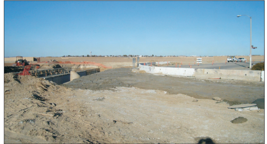
Photograph 2: Looking northeast from the southwest corner of West Ave. J and 65 street at the storm drain construction.
