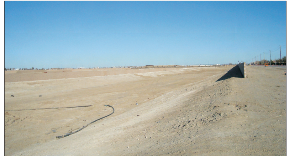
Photograph 4: Looking east from the northeast corner of West Ave. J and 65 street at a new basin that will be incorporated with the storm drains.
