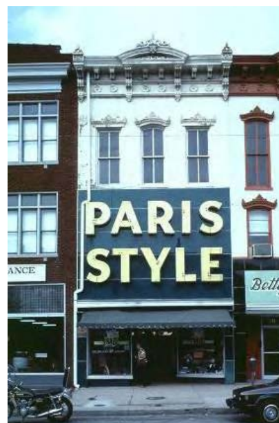
Inappropriate use of signage on facades:
