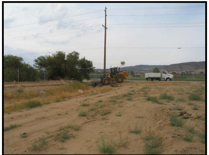
City of Lancaster clearing and re-grading off-site active constructed drainage on July 10, 2007
